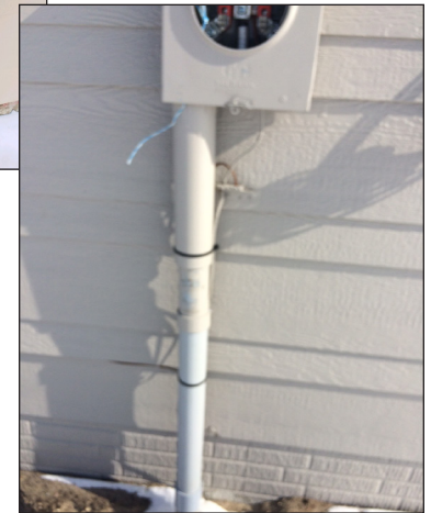
R-3 Expansion/slip riser setting is over four inches.
