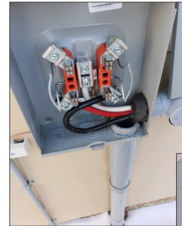
M-3 Riser/cable used knockout too close to home service.
