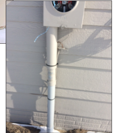
R-3 Expansion/slip riser setting is over two inches.
