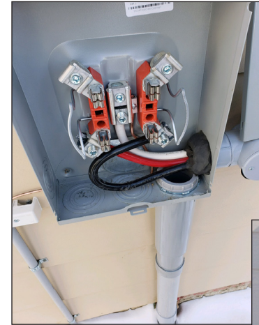
M-3 Riser/cable used knockout too close to home service.
